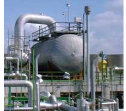
SUPERCLAUS® Selective Oxidation Reactor
