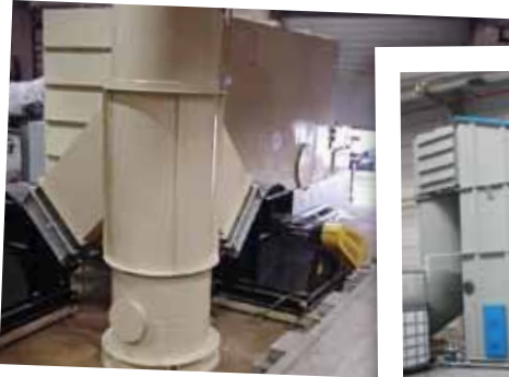
Custom blower module and stack
