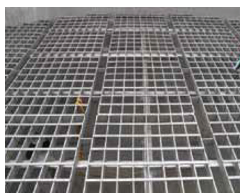
PACKING SUPPORT SYSTEM CLOSE-UP
